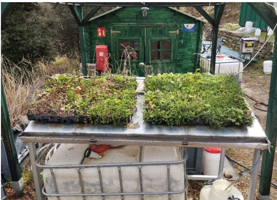
Figure 19: Image of the two Sedum modules of the roof-pilot structure with the IBC tank with raw water and the effluent tank, ready for disinfection underneath (©LEITAT)
